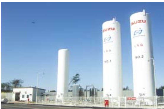
Liquefied natural gas (LNG) plant
