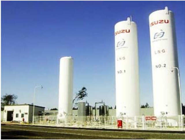
Liquefied natural gas (LNG) plant
