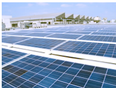
Fujisawa Plant's solar power panels
