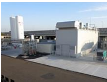
Tochigi Plant Co-generation System
